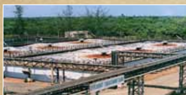
Central Liquid Effluent Treatment plant
